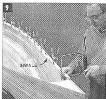
CLAMP THE ASH INWALE to the hull 1/4 in. below the edge, and trim one end to fit. Screw the inwale to the hull, then trim the other end.
